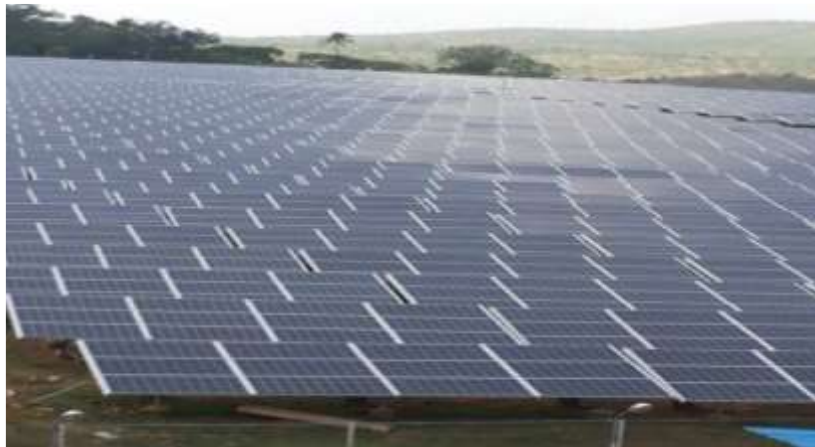
Fig-3: Poly crystalline Solar Panels
