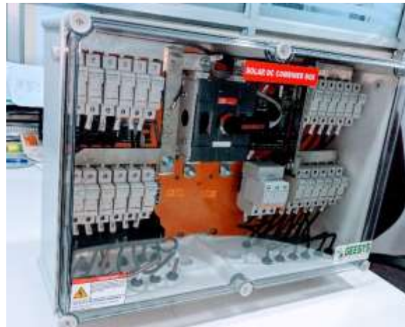
Fig-5: junction box
